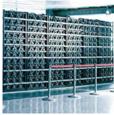
Energy storage system
