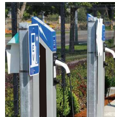
DC charging station
