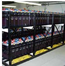
Server power supply
